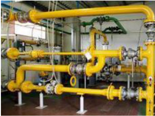
Figure 3: Pressure reduction station.
