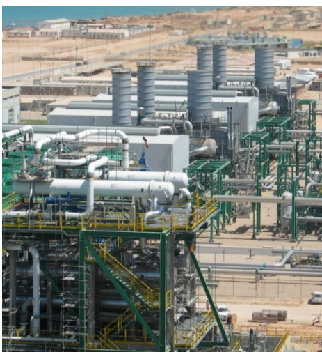
Figure 1: NG compression station.
