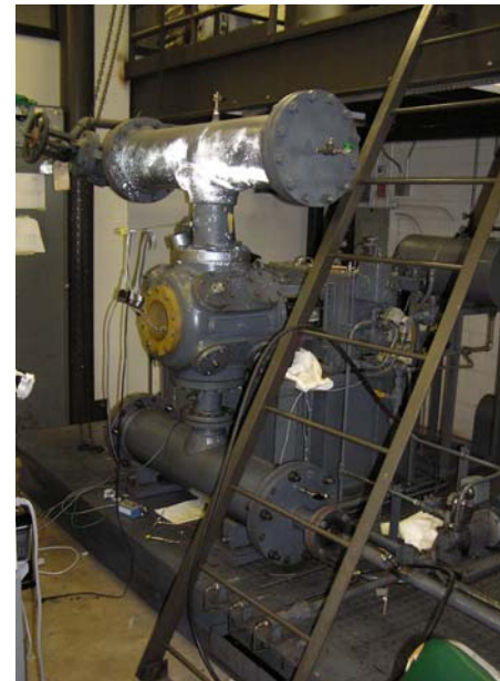
Figure 2-25. Original Reciprocating Compression Test Facility (RCTF) Bottle Design
