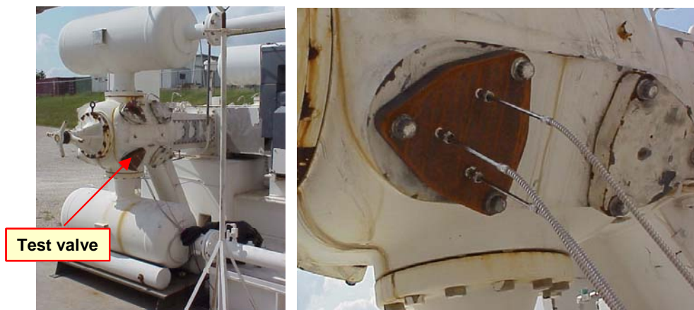
Figure 4-27. Ariel Reciprocating Compressor Used in Measuring Valve Motion (Left) with Optical Position Probes Mounted on Valve (Right)
