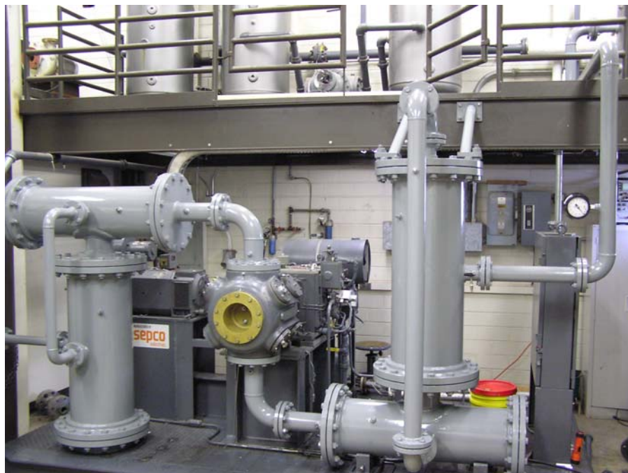
Figure 2-27. Modified RCTF – Two-Bottle Acoustic Filter Design Installed
