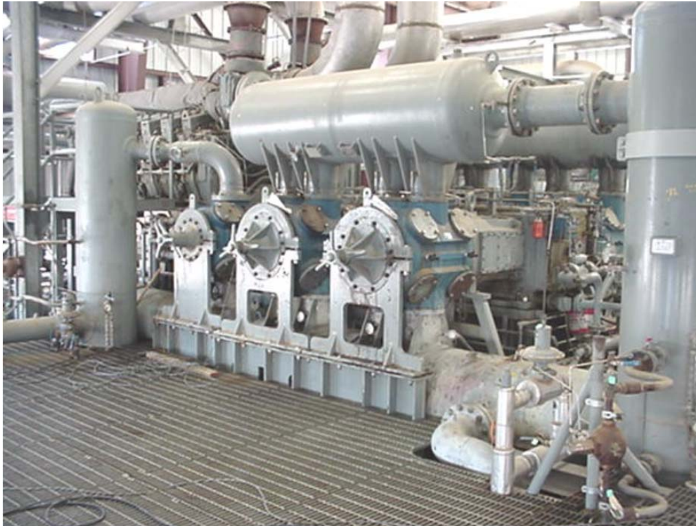
Figure 2-10. Modern High-Speed Unit (2,000 to 3,000 HP) – Unsuccessful Design Required Multiple Gussets to Fix the Design Problems
