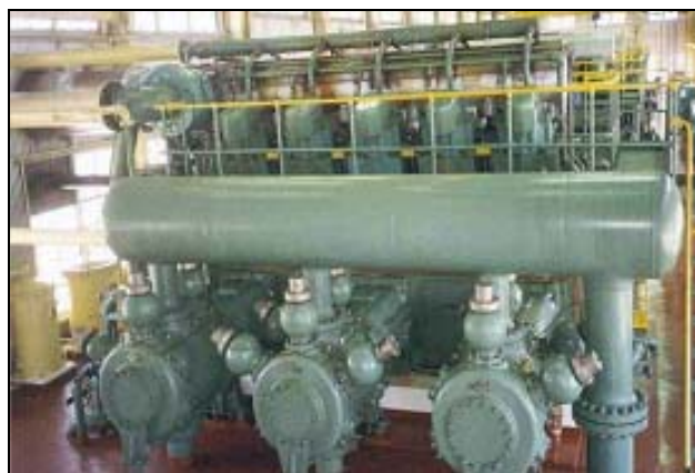
Figure 1-2. Slow-Speed Integral Compression Running at Less Than 300 RPM in the 1,500 to 2,500 HP Range With Pulsation Control Systems
