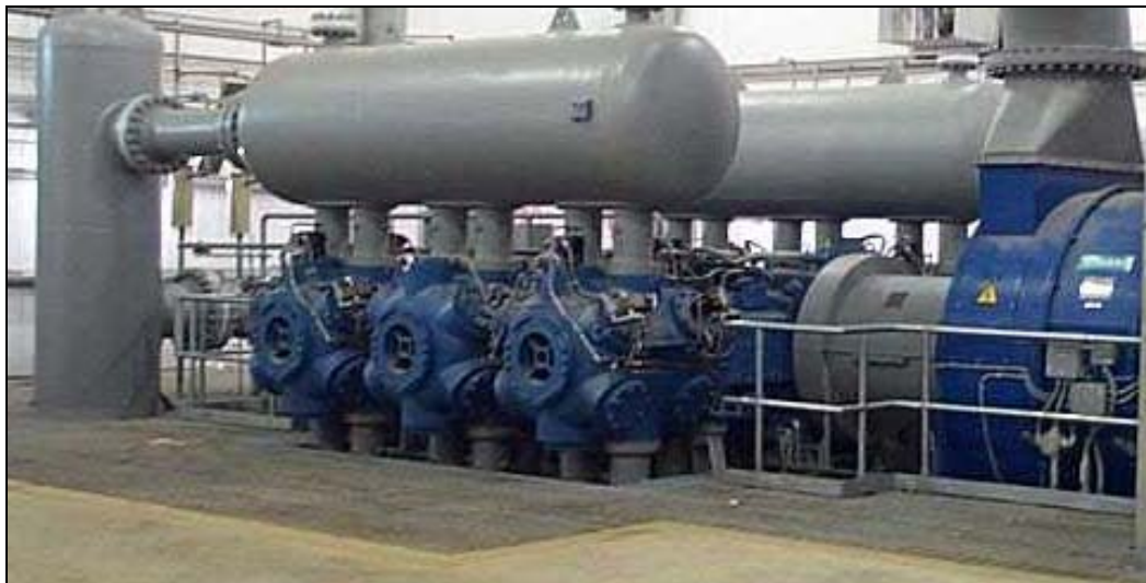
Figure 1-4. Modern Large High-Speed Separable Compressors Running in the 500 to 1,000 RPM Range in the 8,000 to 10,000 HP Range
