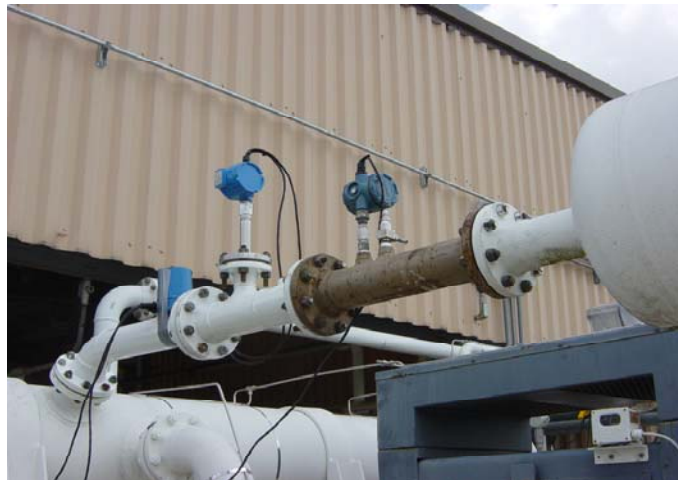
Figure 5-30. Insertion Flange-Mounted Target Meter in Suction Choke Tube at ARCT Test Bed
